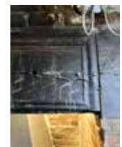
The ogee-edged bressummer moulding along all four edges in the southern room - originally the parlour
