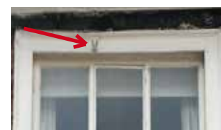
2 St Margaret's Place. Opening light set within a fixed window with a clip above
