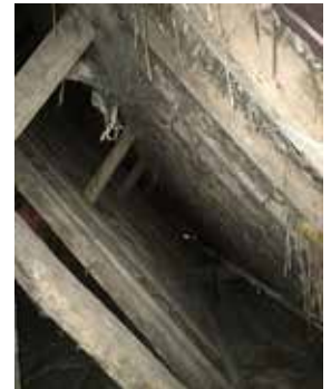
(right) the medieval roof to the left was oversailed by the later roof, thus preserving it
