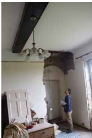
The high ceilings (3m+) of the ground-floor rooms, and one of the many archways into rooms
