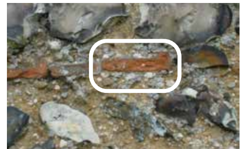
right: A section through a Roman tegular showing its up-turned end which fitted beneath the curved imbrex. found amongst many in the north wall at Coltishall St John the Baptist
