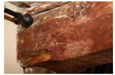
above: remnants of red paint
