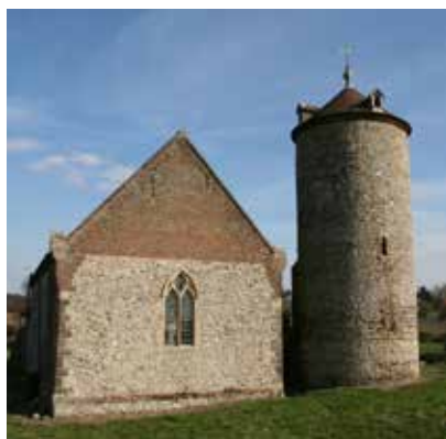
below: The quoins of the rebuilt church and the band of conglomerate in the tower
