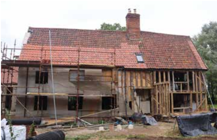
Mardle Hall, south face. The progress of the hempcrete infill (see sidebar) can be seen in the western half
