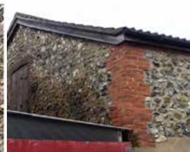
the western gable with small black flints in the darker area, possibly indicating original flintwork
