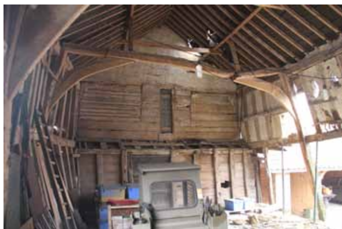
The inside of the barn, showing one of the two broken tie beams that have pushed the wallposts outwards
