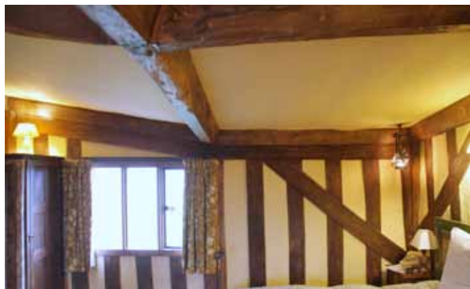
The parlour chamber - the wall-plate showing the amount of sinking at the parlour end
