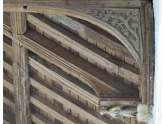
One of the spandrels beneath the tiebeam for the queen posts and the false hammer beam, with angel, behind it
