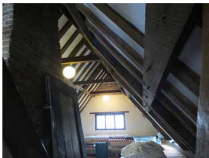
Below: The roof of the Row 111 House, mostly resulting from the eighteenth-century alterations
