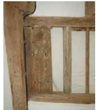
Shutter with auger holes
