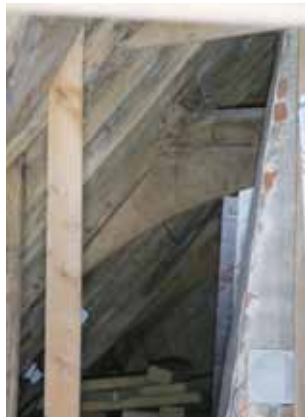
Part of the large curved brace of the roof over the hall chamber
