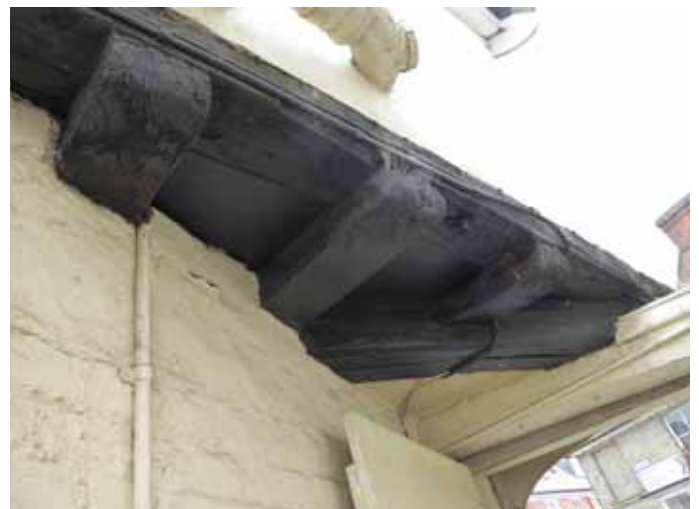
Jetty and Dragon beam originally facing the marketplace, now above a narrow alleyway between buildings (photo Anne Woollett)
