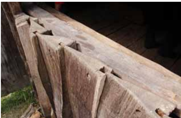
feathered riven boards fitted into grooves in their neighbour to keep out the weather
