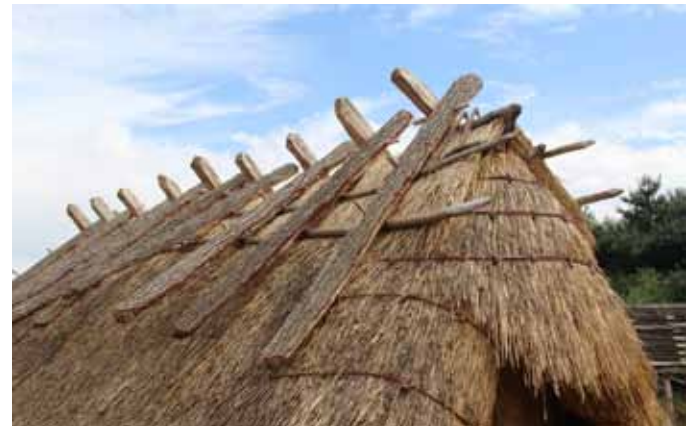
Timber beaks along the ridge to anchor the thatch, as seen in Denmark
