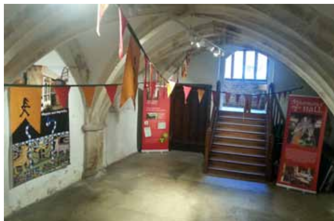
Is the moulding on the capitals in the undercroft contemporary with the occupation of Ralph de Middleton around 1320?
