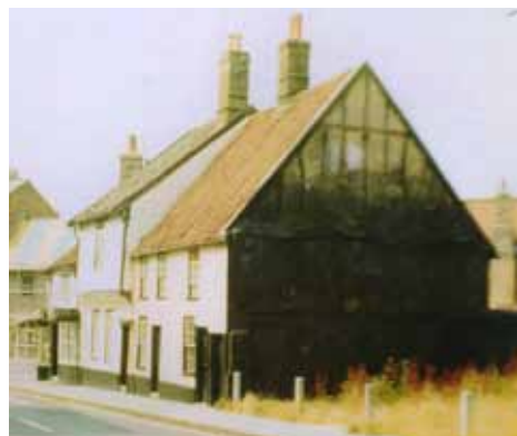
The burnt external wall in the 1980s
