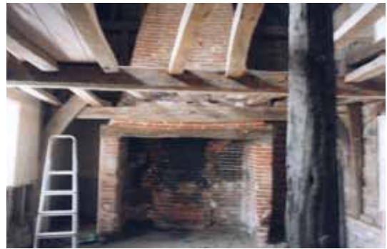
The brick stack built within the medieval smoke bay. Support for the inserted floor is behind the arched braces (photo: Mo Cubitt)
