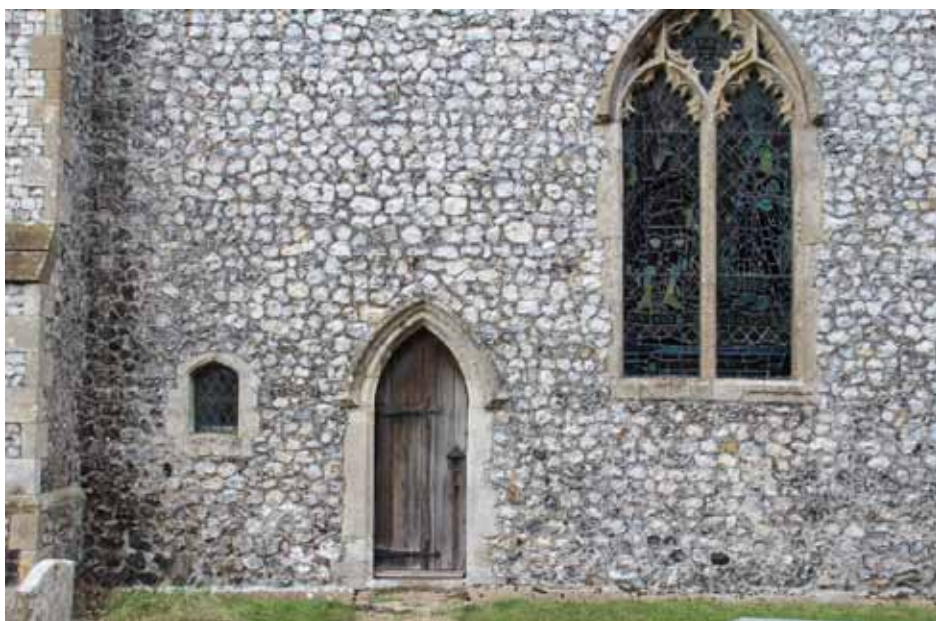
There has to have been a reason for such a small opening in such an odd place - here at Aldborough St Mary, seen from the outside.
