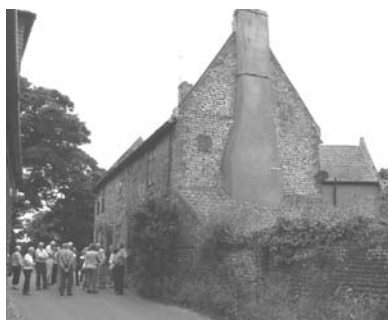
Fig. 2 Dyer House (a) external stack on flint gable with two blocked windows.
