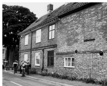
(c) south facade: note two levels of string courses and blocked windows.
