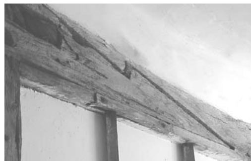
Fig. 3 A stop-splayed and tabled scarf with under-squinted abutments, transverse key and four face pegs; this scarf is capable of resisting every known stress: hog, sag, torque or winding and flexure. In use from c. 1250. A similar joint (below) is to be found in Wingfield College. (Cecil A. Hewett, English Historic Carpentry , Phillimore & Co. Ltd, 1980)
