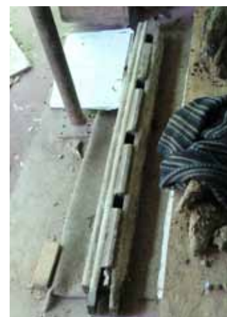
Moulded window head removed after being uncovered in the front wall of the parlour as part of recent restoration. (It has been replaced in situ)
