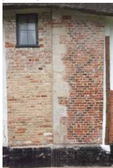
Different brickwork on the two wrap-round gable ends associated with the two stacks
