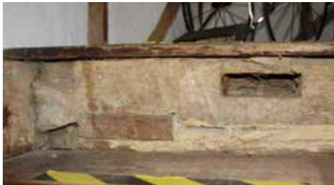
The re-used tie beam, on its side, showing the characteristic half-dovetail joint to the left that enabled it to grip the wall plate in its original location
