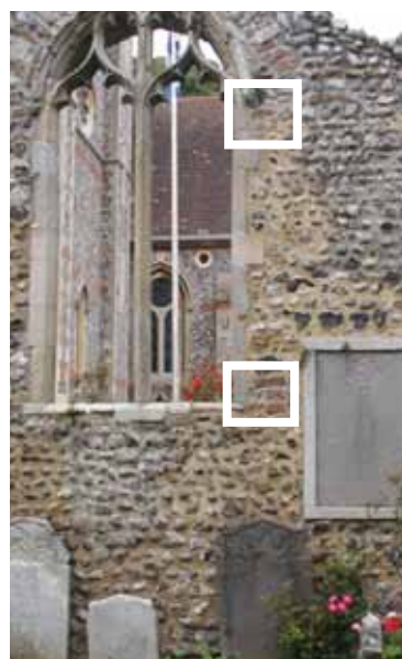
put-log holes too close to the window for it to have been the original one
