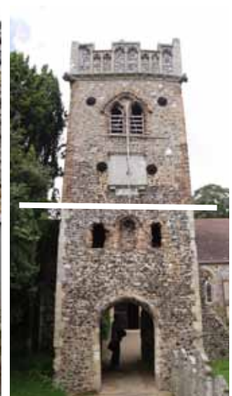
tower extension with brick quoins, built above a two-storey porch with stone quoins
