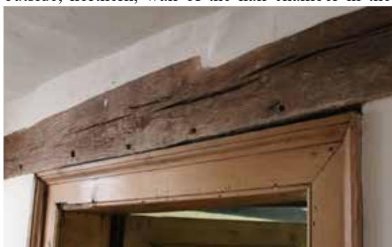
Five pegholes in the wallplate for a window in the hall chamber (seen from the outside)
