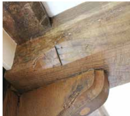
The applied additional supports at either end of the principal joist in the hall
