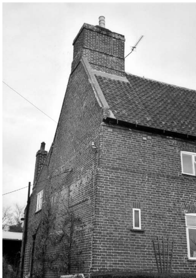
Spa Farm. Enigma of six flues for two internal fireplaces; could they indicate possible lost outbuildings at ground floor level?
