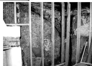
First floor: Tie beam and brace in front of stack—wall plate and ?window on south wall. Wattle and daub infill.
