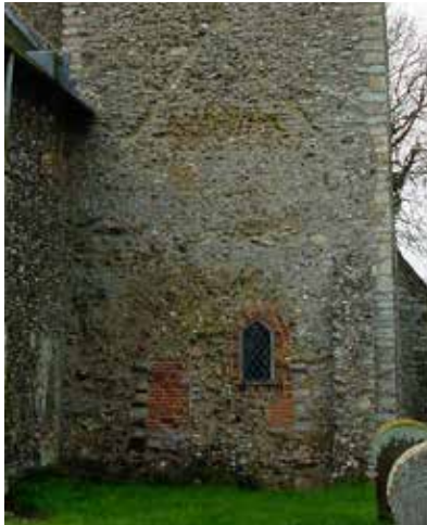
Roof scar of the original chancel in the tower wall, with bricks partially filling the old chancel arch
