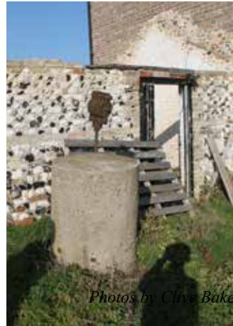
This heavy concrete block is part of the electricity generating system for the house
