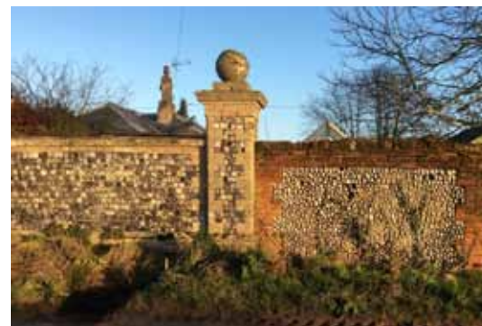
The multi-period flint boundary wall, parts of which require significant repair work
