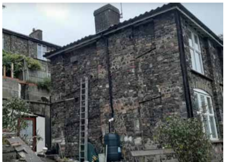
The end wall of St Leonard's Terrace built with the waste bricks, with St Michael's Terrace above
