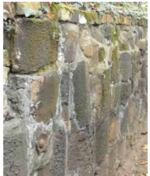
Curved pieces of lining built into the wall up to Kett's Heights, including one of the anchoring bolts
