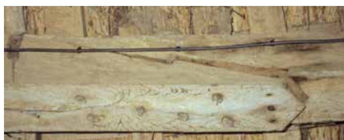
Plate 2 Splayed & tabled scarf with transverse key & sallied square abutments in north-arcade plate
