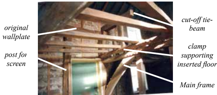
Photo 1 (both by Mo Cubitt) The hall/service room frame and door in the front wall
