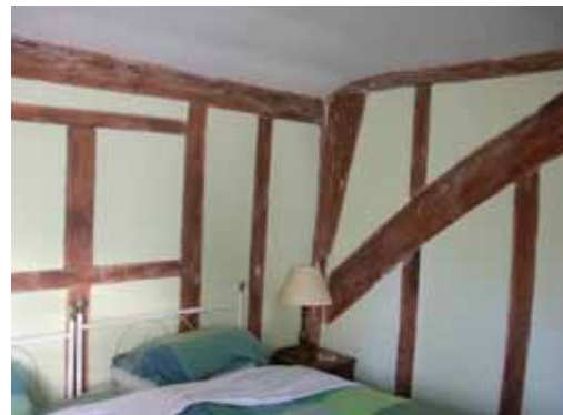
Substantial framing upstairs with one of the eighteen braces in the house
