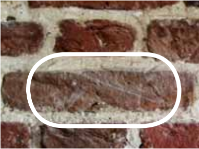
Skintling marks (defined overleaf)
