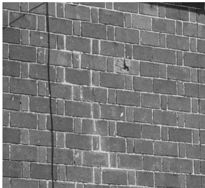
Small cottages at the top of Mount Street with a version of rat-trap bond.
