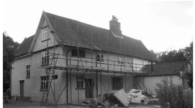
The Old Post Office, Gissing, under scaffolding but making progress. The range to the rear is a modern, timber-framed extension. The wood for this extension was selected by our guide to Great Bradfield Woods, Andrew Moore.
