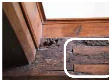
Filled mortices after the re-location of the principal joist to allow sufficient headroom above the new staircase (photo Ian Hinton)
