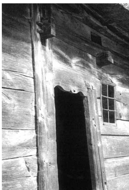
B - wall planks grooved into uprights. Above the door are two more examples of the anchor-beam, or tusk-tenon, discussed in Newsletter 20
