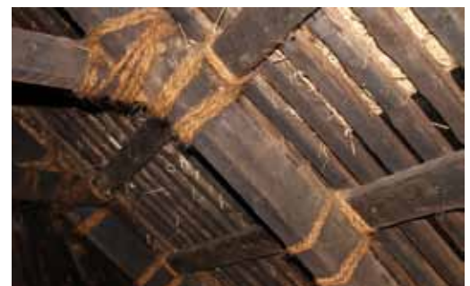
Hebridean roped joints in the black house, with the heather undercoat poking through
