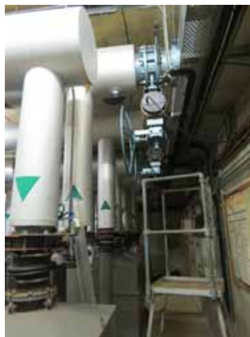
part of one of the many plant rooms underground
