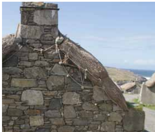
Twentieth-century gable end, requiring wooden pegs to anchor the ropes after the hipped-end and its crow post was replaced
