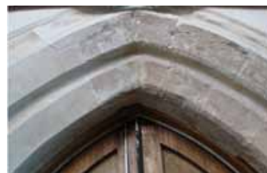
Fire-discoloured stone in the chancel north-door arch
