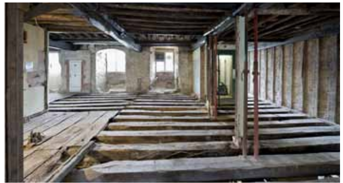
Buttery: view northwards, showing massive floor joists and east wall studs (right), all of 1382-3.
