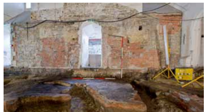
The uncovered stone arch of the original fireplace in the kitchen, later filled in with brick
