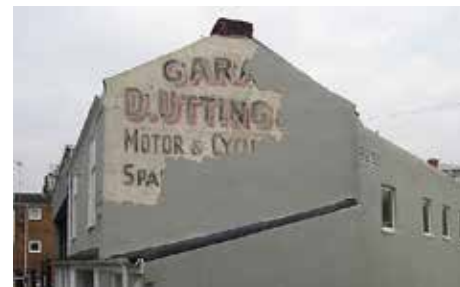
The remains of an advert in Dereham Road after repairs to the wall
