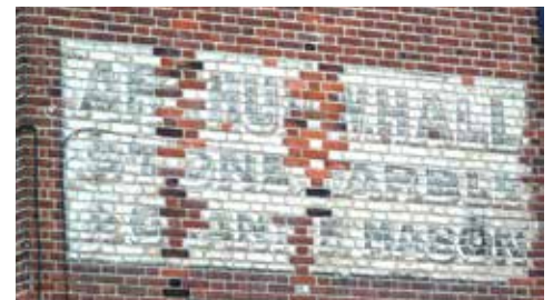
Below: Remnants of a sign in St Augustine's St, showing later brickwork repairs
