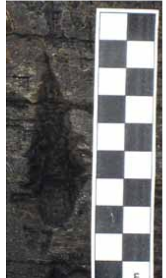
figure 7 - burn mark on the chimney bressumer (photo John Dean)
