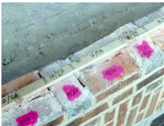
Numbering the bricks of Longport Farmhouse. The brick positions were also recorded on a wooden battens...
