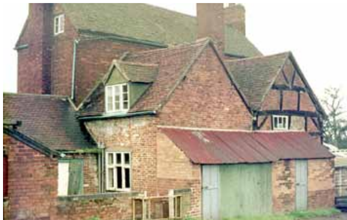
Monkspath Hill Farm before dismantling. The two matching gables reflect the form of the original C17 “M” roof.
