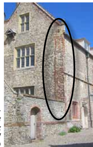
Figure 4 - Toothed brickwork in the south-east corner of the west range, still awaiting the extension after 433 years! (photo Rosemary Forrest)
