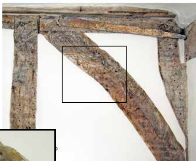
far left: the section through Friday Cottage showing the nailed-in partition and the missing stud in grey
