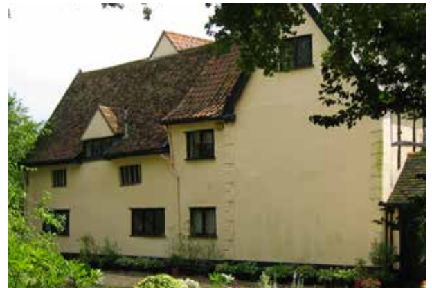
Most of the Arts & Crafts work was removed in the 1960s necessitating the replacement of most of the ground-floor studs in this wall and revealing the unglazed first-floor windows
