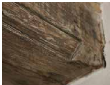
Sunk-quadrant chamfers to the principal joist both upstairs and downstairs in the crosswing
