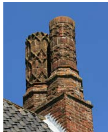
Old Hall Farm House, Foulsham: east chimney stack. Did the stack give function or symmetry? It was not possible to find matching hearths inside the house.
