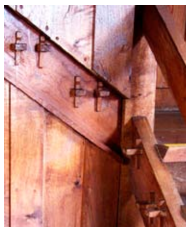
Parkes Castle, Co. Leitrim where anchor pegs have been used in a restored building which are both decorative and useful. Parkes Castle dates back to the 1100s but was extended in the early seventeenth century and restored in the twentieth.
