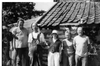
Karen Mackie showing Dirk Bouwens how to 'butter' clay lump; Dirk turned up to lay final clay lump after students had rebuilt wall; Dirk applying render to clay lump. Note how skilfully repaired wall is contoured for authenticity; Master builders and Dirk posing in front of their handiwork. (Photos: Roger Crouch)
