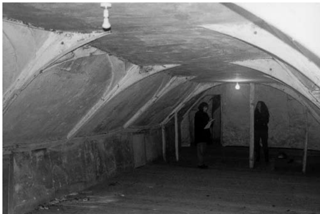
High arch braces to an upper collar and large section windbraces to butt purlins. (photo: Michael Brown)
