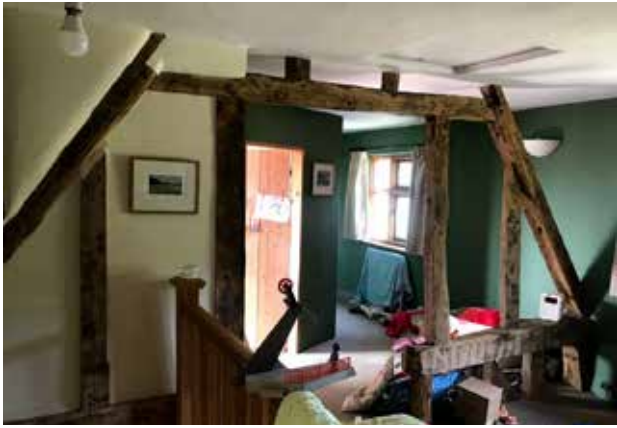
The original end wall of the house, showing the steep roof and position of the gable end window
