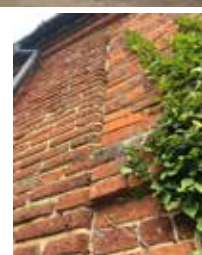
the join between the gable and the later bricking-up (photo Les Scott)
