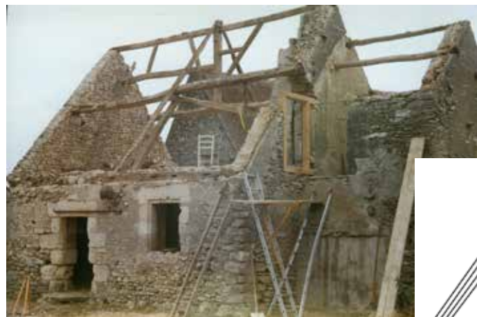
above: during the roof replacement the previous year - an interesting mix of truncated principal rafter and king-post construction
