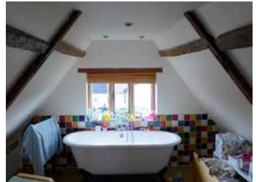
The shaved purlins in the roof of the pantiled extension
