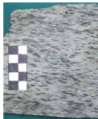
Close up of the decorative schistose slate from Norway on the chancel roof
