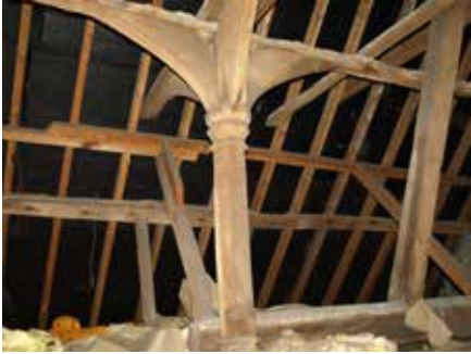
(left) Crown Post roof - before c1500. Higher status - meant for display in the roof of an open hall (the side purlins here are later insertions), or in upper chambers. If smoke blackened - open hall, if clean (as left) open from a first-floor chamber.
