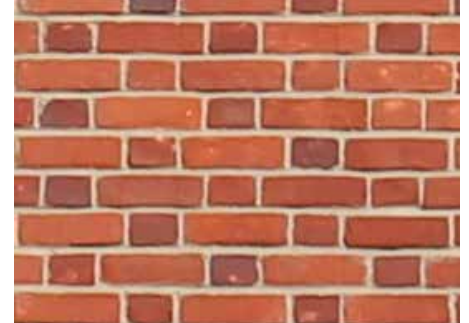
Flemish bond - almost always post 1650. Each brick has the opposite sort on every side, so headers and stretchers alternate, both horizontally and vertically
