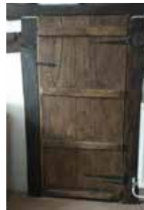
simple ledging with no diagonal bracing
